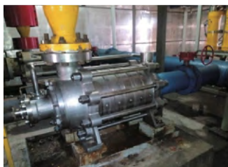
图7 HSB220/620 海水淡化高压泵现场运行 Fig. 7 HSB220/620 seawater desalination high pressure pump is in operation
